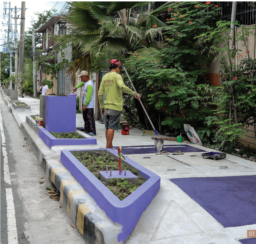
01 On-going construction of the Green Open Reclaimed Access (GORA) lane project which aims to promote walkability
